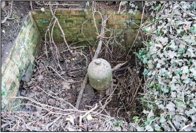
The derelict ram pump at Alwalton in its chamber today. It is no longer in working order and the pump building has been demolished (Author).
