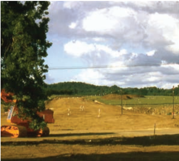
Work on the new road is well under way in July 1975 (Richard Adams)
